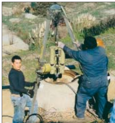
Technicians with The Lighthart Corp. set up at one of the manholes along the route from the Loyola Marymount campus to the main city sewer.
