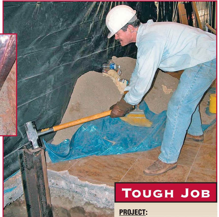
A technician drives in an I-beam as part of the foundation for the pull.
