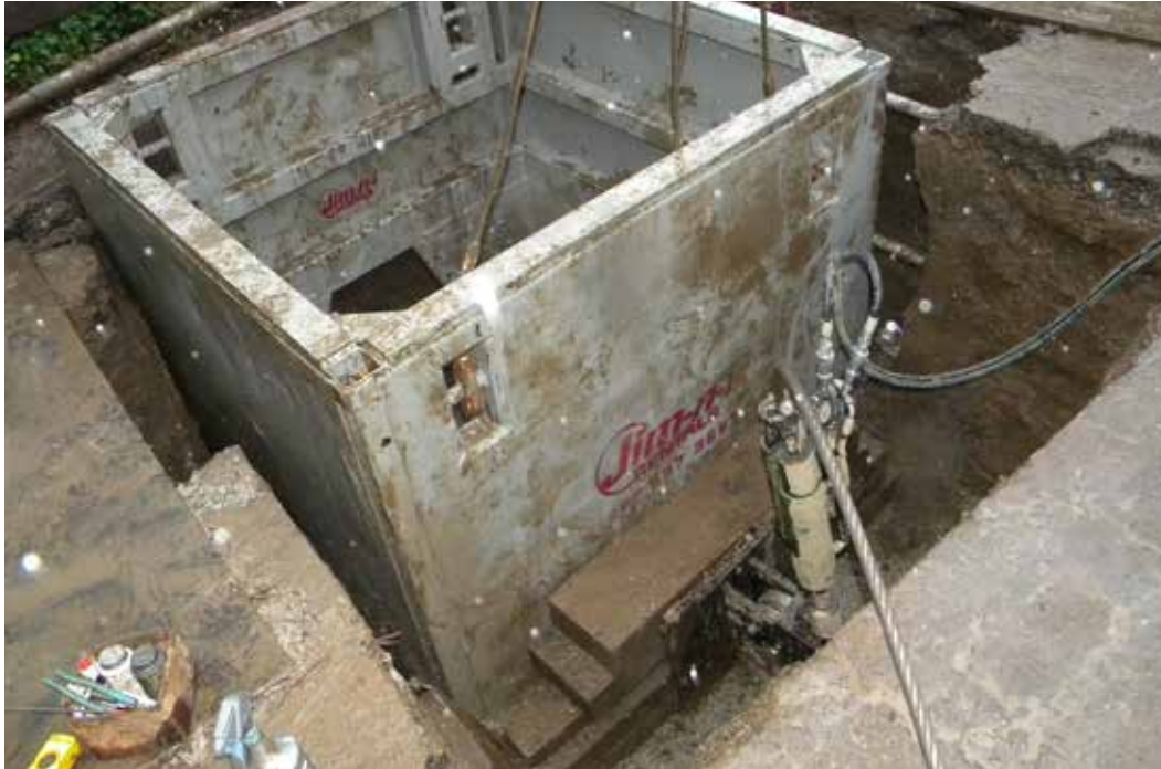
Figure 8 P51 with manhole box
