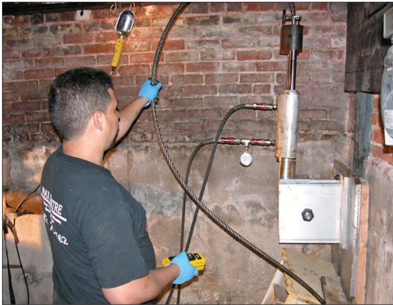
A static lateral bursting system pulls a 4-inch sewer into a basement.
