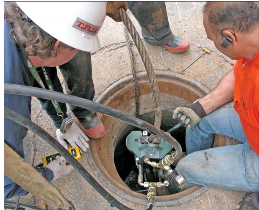
A 60-ton static puller uses 1-inch cable to burst an 8-inch clay sewer main. (Photos courtesy of TRIC Tools Inc.)
