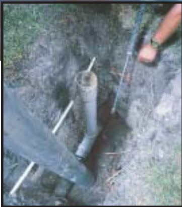
During lateral replacement, cleanouts are installed every 75 feet to comply with city codes.
