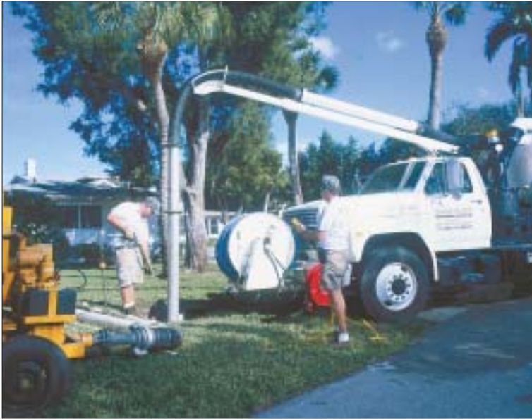
Entry pits for pipe bursting are cut with a water jet, then vacuumed by a Vactor truck.
