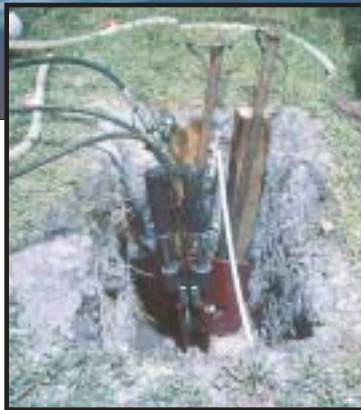
The small hydraulic puller used in Sarasota's pipe bursting project generates up to 60,000 pounds of pulling force.
