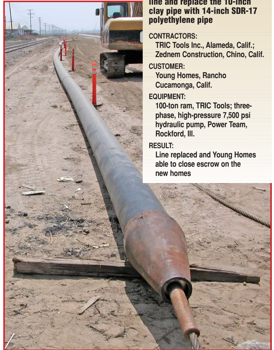
A 360-foot length of polyethylene pipe is attached to the bursting head and ready to pull.
