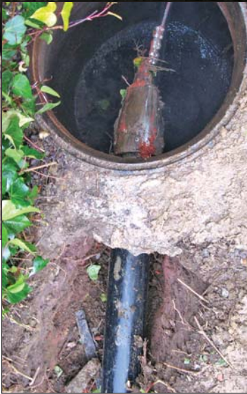
A pipe bursting head emerges from a manhole after a 350-foot run. Stege Sanitary makes pipe bursting a major part of its pipe rehabilitation program. (Photo courtesy Stege Sanitary District)
