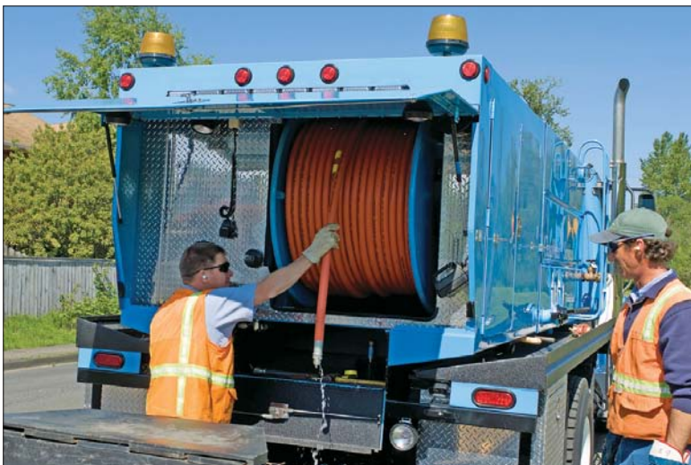
Crew lead Bob Sorenson and field construction maintenance technician II Jim Stahly prepare for a pipe cleaning job.
