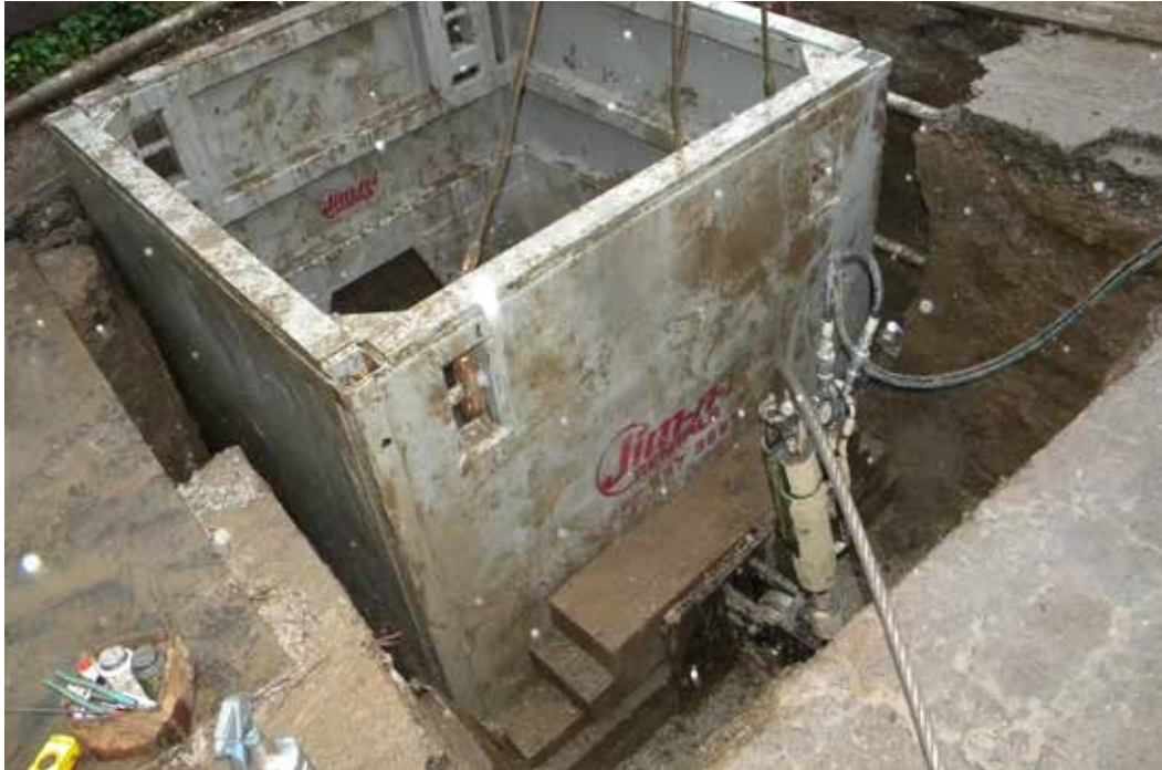
Figure 7 M50 with manhole box
